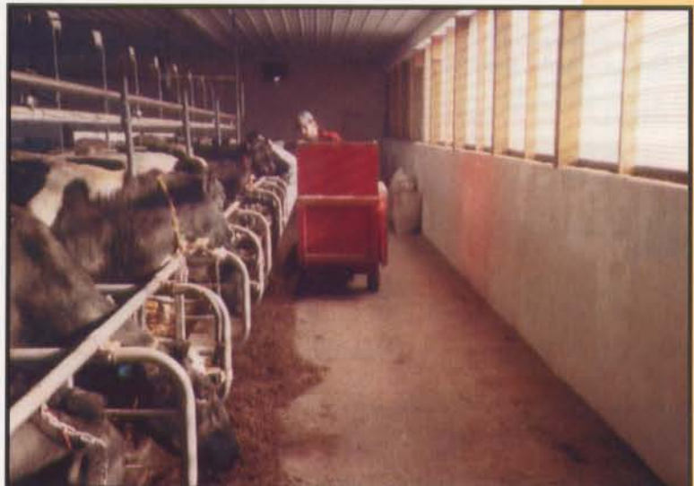
This tie stall barn is on the Tim Easton Dairy in Genesee, PA. The POLY VENT is in the closed position.
